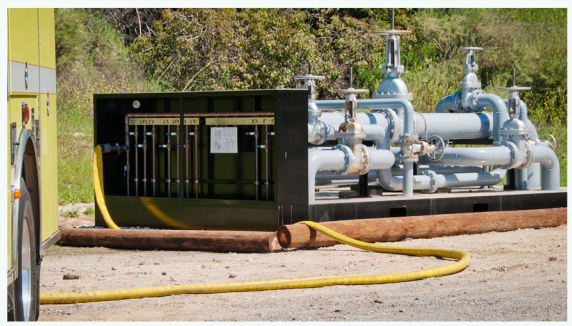
PUMPER SUPPLIED DISTRIBUTION MANIFOLD
