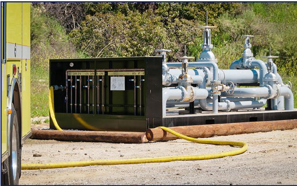
PUMPER FED CONTROL VALVE MANIFOLD AND PIPING ARRAY
